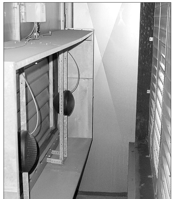
Probes Mounted Before a Damper
